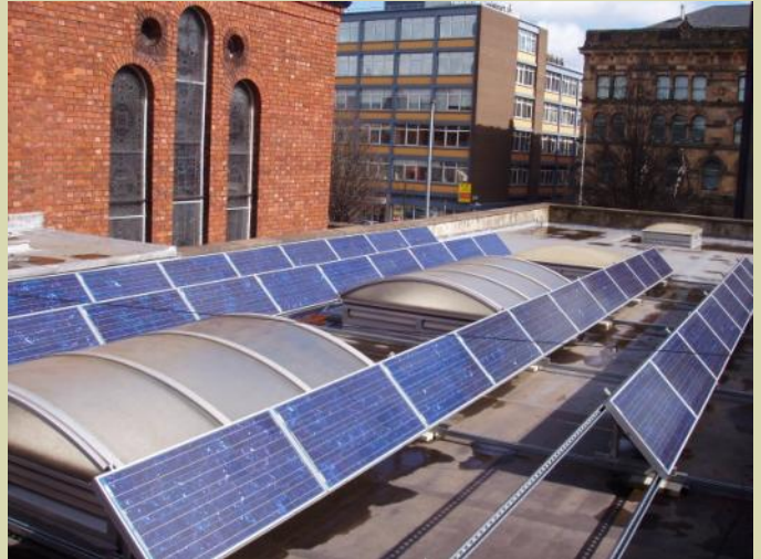
Photovoltaic panels on the roof of St George's
