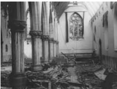
The west end side aisle in St James' after the bombing. The black curtains on either side of the window were to prevent interior lights revealing the location of the church at night.
