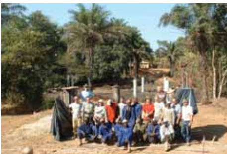
FIA volunteers building a Bailey bridge in a remote village where the river often flooded in the wet season.
